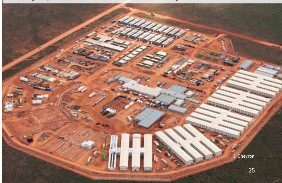
Taking shape ... an aerial view of the Construction Village on Barrow Island.
