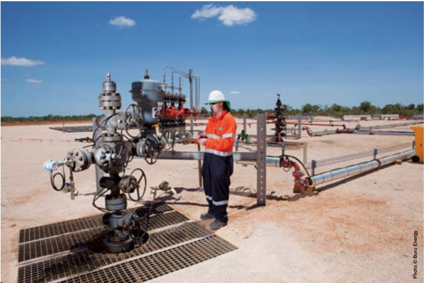
Ungani 2 wellhead and Buru Energy field operator
