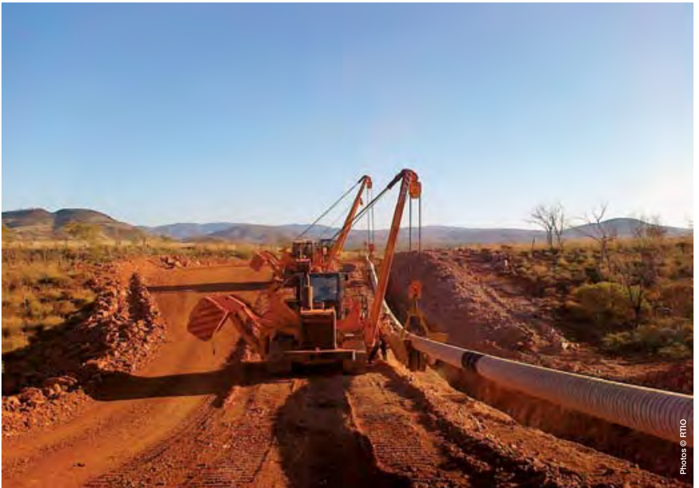
Top left: Close up of the Deckhand®. Top right: Lifting the pipeline into place. The Deckhand® has helped lay 85 km of gas transmission pipeline. Bottom: The West Angelas petroleum (gas) pipeline will transport gas from the Goldfields Gas Pipeline to Rio Tinto's new gas fired power station in the Pilbara
