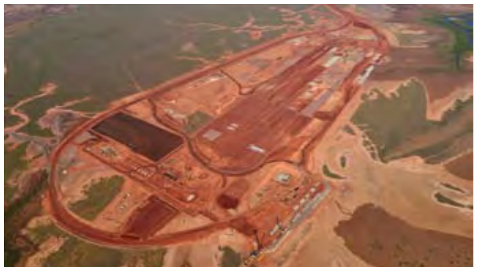
An aerial view of construction of Roy Hill's Port Rail Loop and Stockyard facilities.
