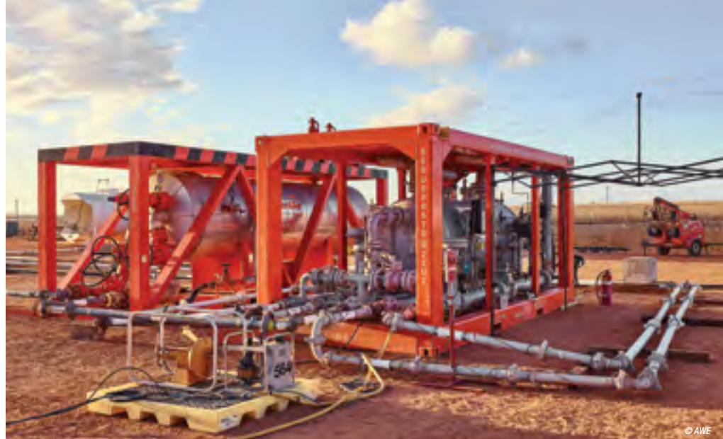
Irwin-1 is the first well of a three-well drilling program planned for Perth Basin in 2015.
