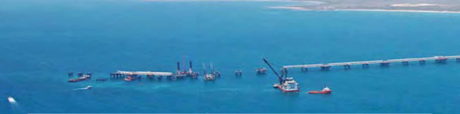
Work continues on the 2.1km LNG jetty, with all 56 jetty caissons now in position.
