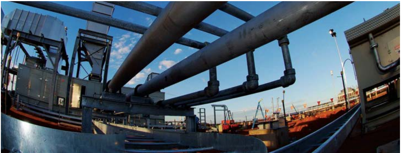
The Dampier to Bunbury Pipeline. Photo: DUET
