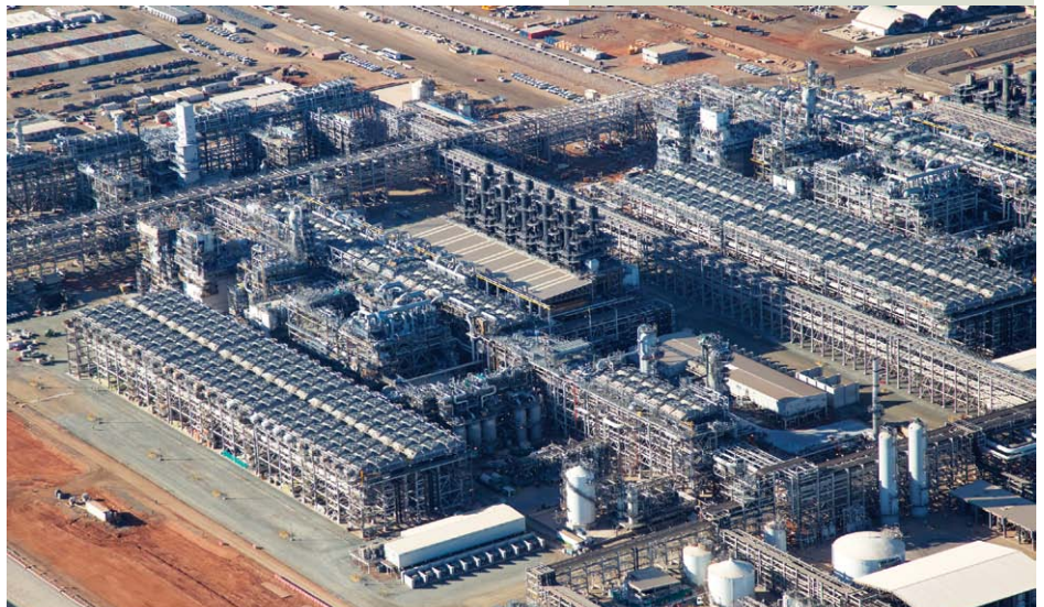
The Wheatstone Project is one of Western Australia's largest resources projects. Photo: Chevron
